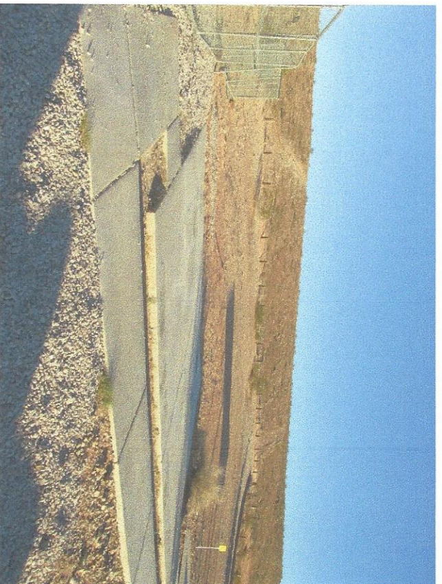
Similar to first photo, this shows where concrete needs to be added; if existing concrete cannot be used, it will be replaced.
